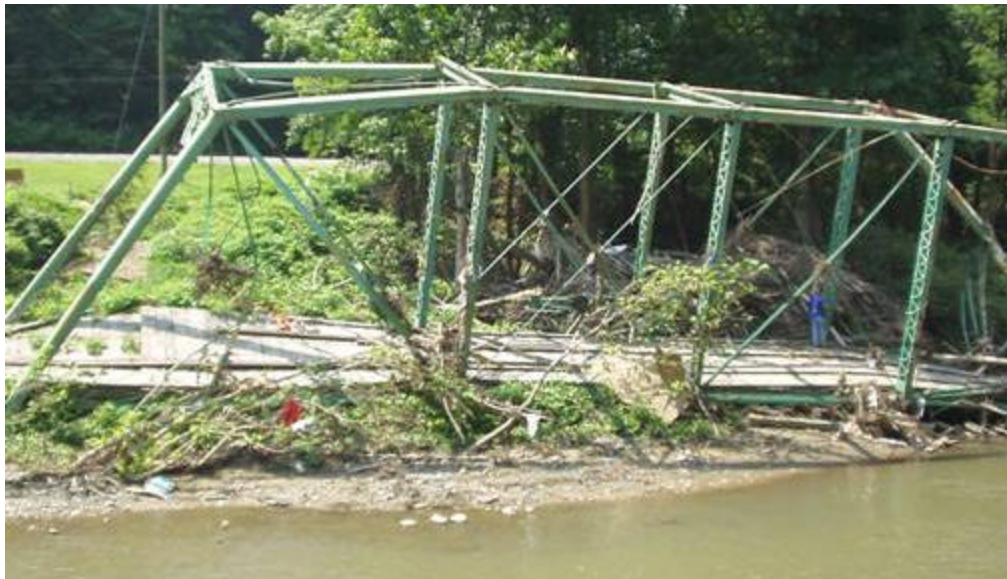
Figure 1-3. Example of Transportation Damages in July 2001
