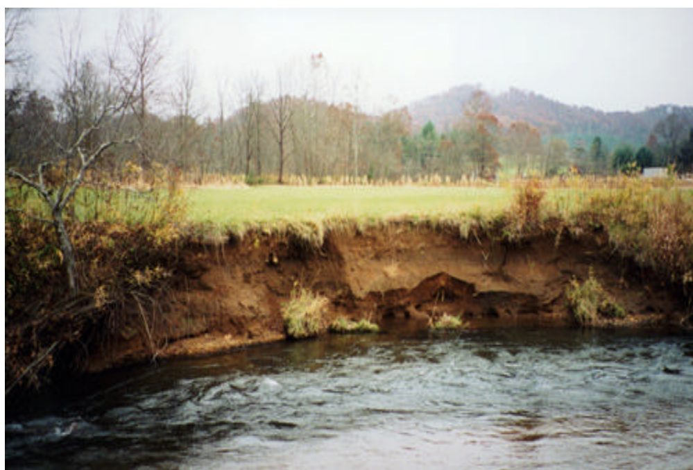
Figure D-3. Damaged Stream Banks
