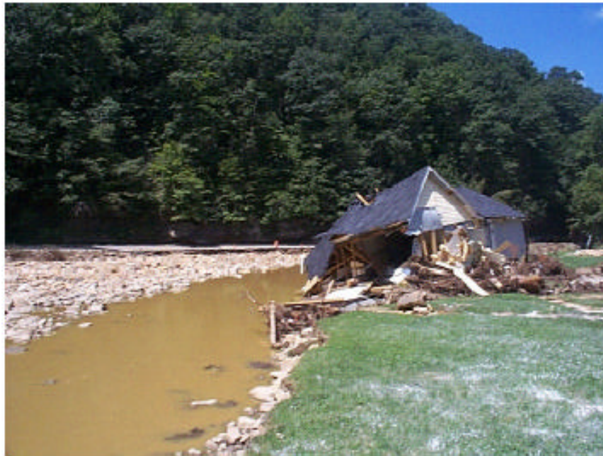
Figure L-1: Residential structure damaged in floodway.
